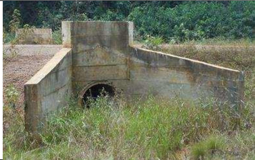
Existing drainage structures along the Buchanan–Cestos corridor showing reinforced concrete and culvert drainage systems, some of which are partially obstructed by vegetation and sediment, potentially affecting water flow and aquatic habitat conditions
